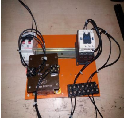
Damper Control Wiring
