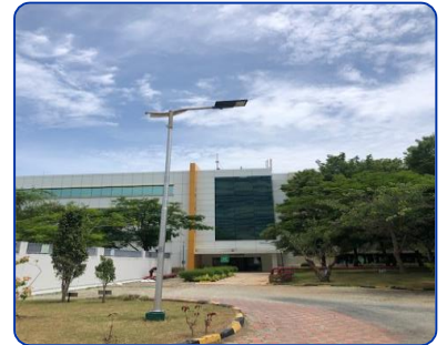
250W MH Street Light to Solar Fixtures
